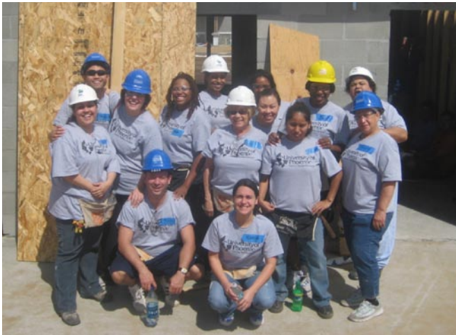
Central Florida staff volunteer with Habitat for Humanity in March to build a home for a local family in need.
